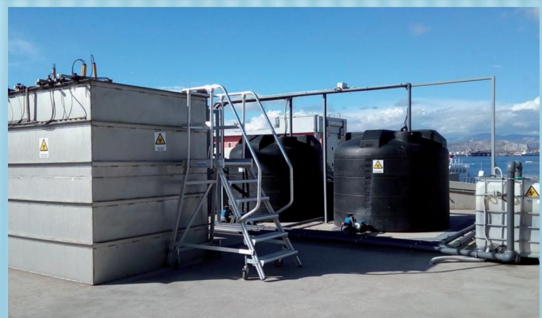
Figure 5. SMARTech4b pilot plant at Psytalia
